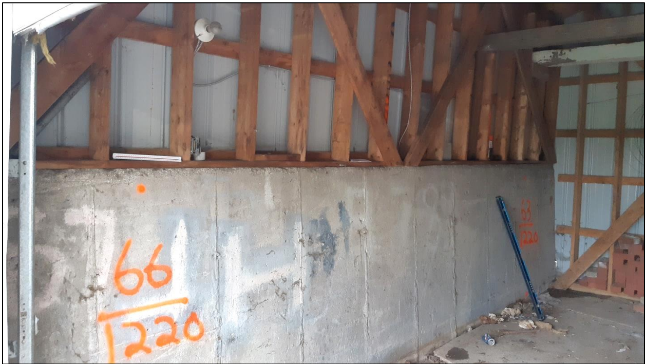
Cracked Retaining Wall – Olympia Room
